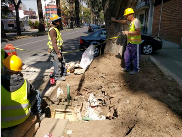
Figure 5. An example of maintenance work performed within the Critical Root Ratio (CRR) destroying part of the root, weakening the anchorage of a specimen and increasing the risk of tree failure. The species, a Jacaranda Mimosifolia , is a common species in Mexico City (CONABIO, 2012).
