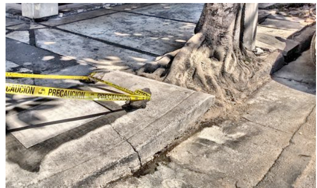
Figure 2. Example of damage and space conflicts caused by proximity of tree roots to urban elements, including pavement cracks, sewer system, electric poles and electrical pit damage. The tree species correspond to Ficus elastica , a common species in Mexico City (CONABIO, 2012).
