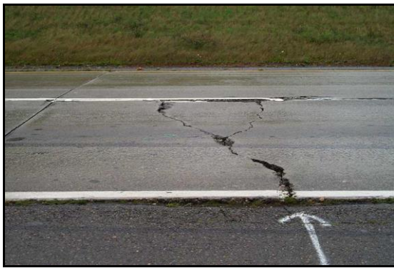
Figure 2. Crack formation on the road (Movea, 2013)
